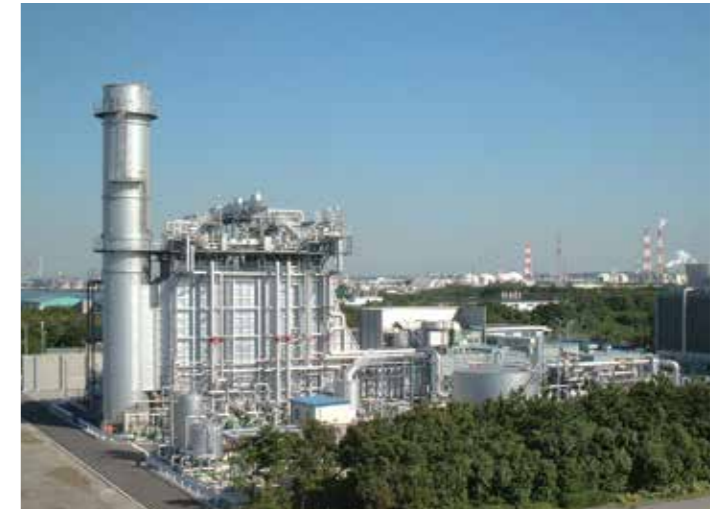
排熱回収ボイラ(横型自然循環式) Heat recovery steam generator (Natural circulation type)
