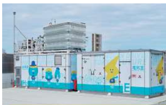
P2G system with water electrolysis equipment for Keihinjima No. 1, Tokyo
